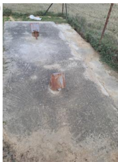
Figure 4-47: Anaerobic pit at Adelaide abattoir close up
