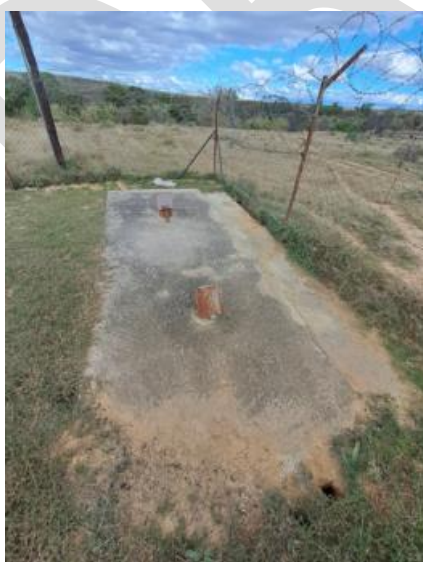
Figure 4-46: Anaerobic pit at Adelaide abattoir overview
