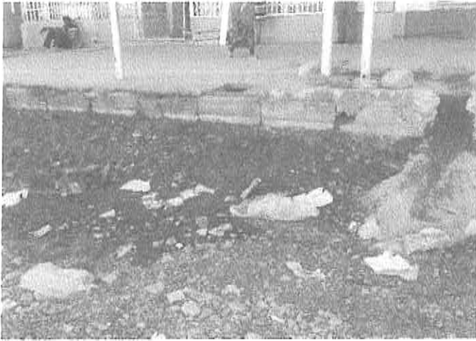
Campbell Street: Box Cut - Water discharged from premises into street
